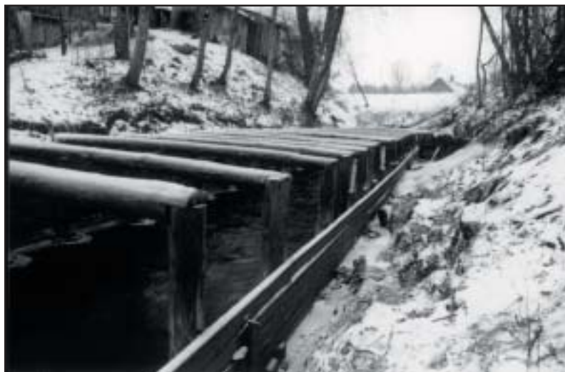
Jugla - canalised river, coming from the hydropower plant. Photograph by Janis Brizga
